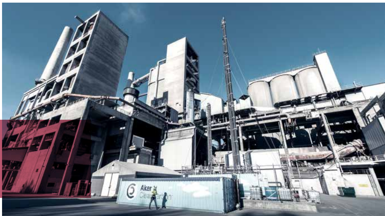
Norcem-Aker Solutions test module for CO 2 capture. Photo: Gassnova
