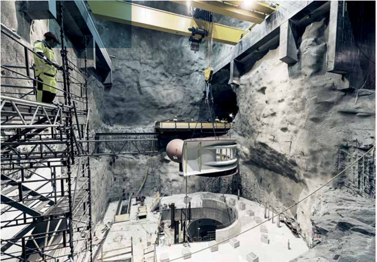
Installation of new spiral case at Iveland hydropower plant. Photo: Agder Energi
