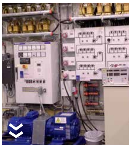
Prosjekt: SmartGrid – National Smart Grid Laboratory & Demonstration Plattform
