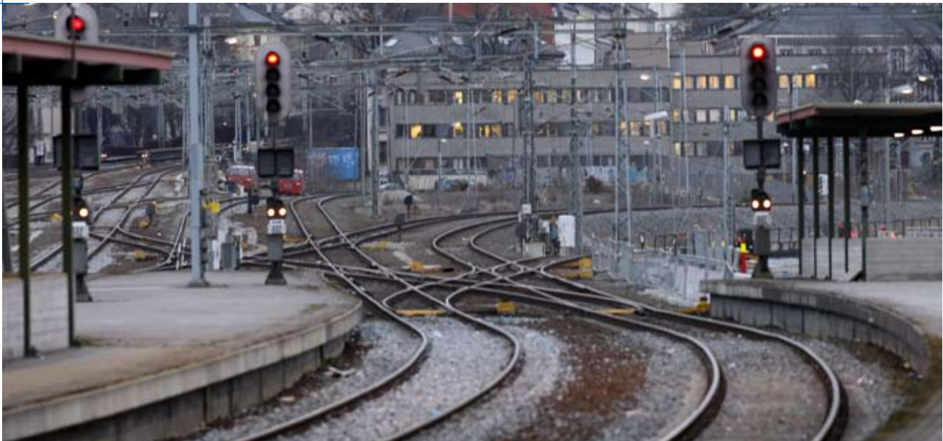
A cable fire in 2007 at Oslo's central train station led to an electrical shutdown, bringing all railway traffic to a halt. Thousands of subscribers also lost access to the Internet. (Photo: Morten Holm, Scanpix)
